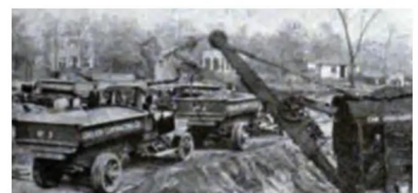
Udelson Contracting's Marion steamshovel and battery of Acme 5-ton trucks, circa 1920 in Cleveland, OH.
